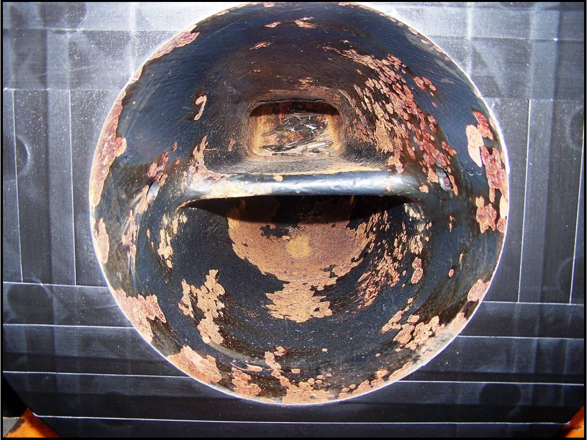
Picture 7 - Cavitation damage to the original surface coating before shot-blasting
