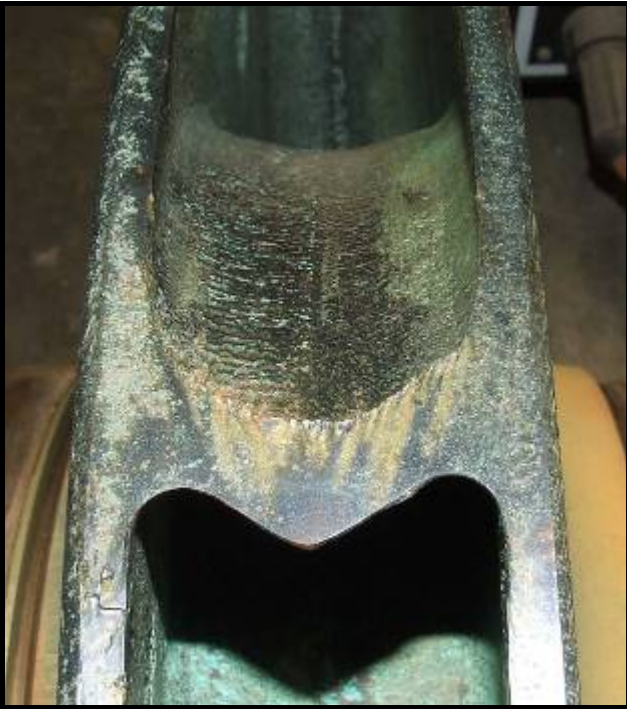
Picture 4 - Discharge vane tip of pump impellor
