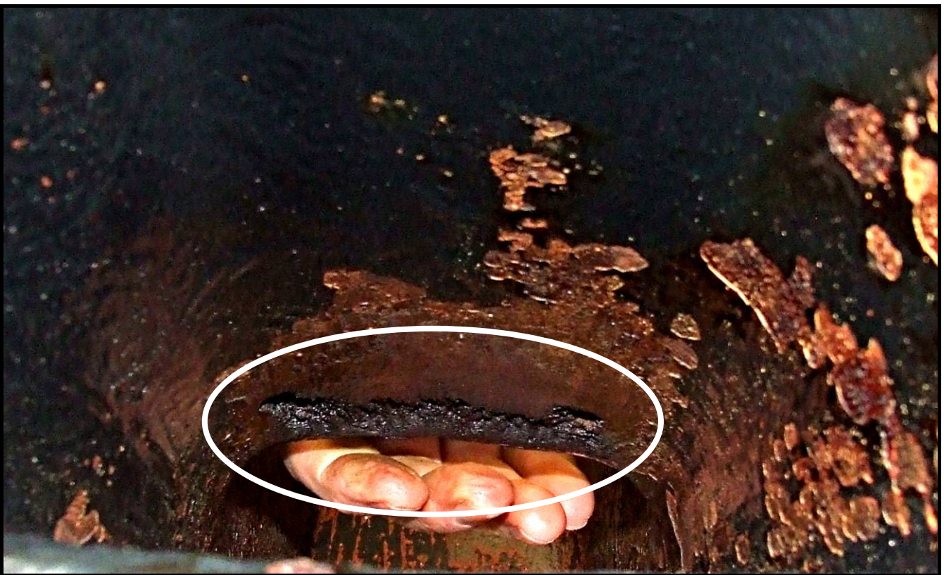
Picture 6 - Cavitation damage to the volute wall
